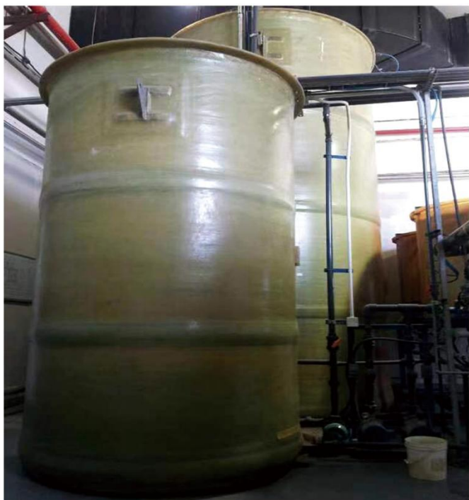
硫酸槽 Sulfuric acid tank
