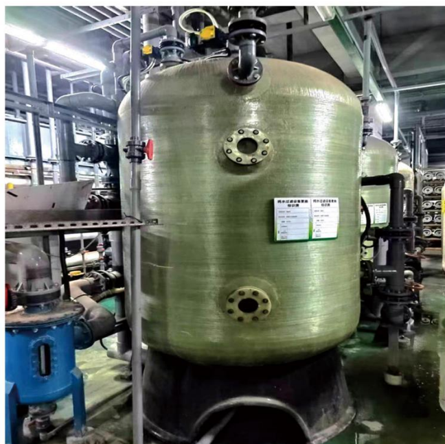
混床罐 mixed bed tank
