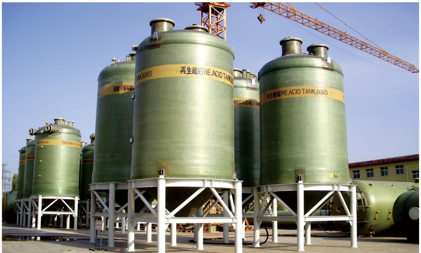
再生酸罐 Regenerated acid tank
