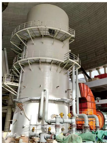
净化塔 purification tower
