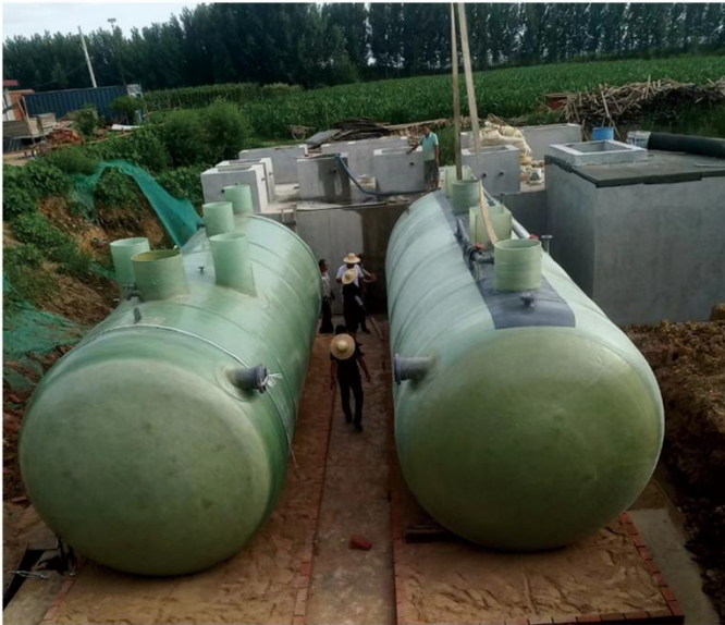
地埋玻璃钢罐 Buried fiberglass tank
