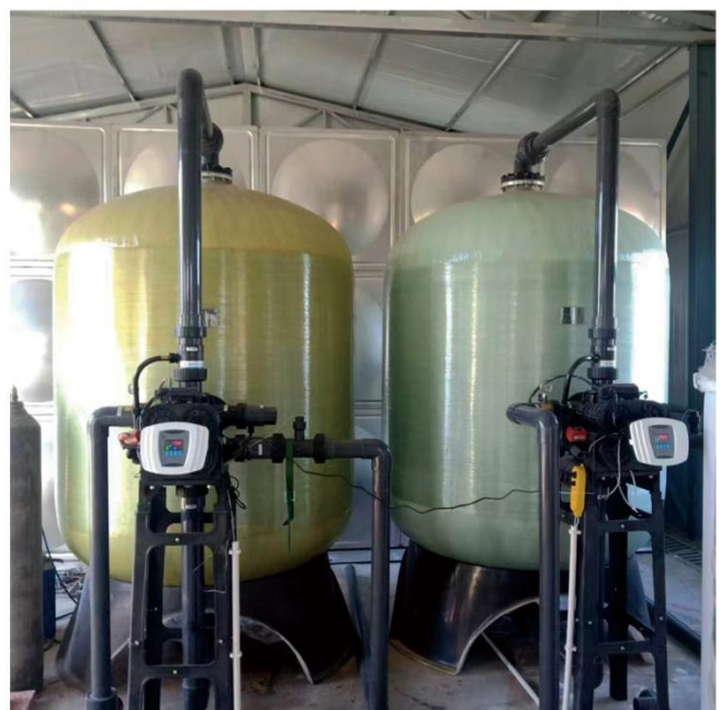
软水罐 soft water tank
