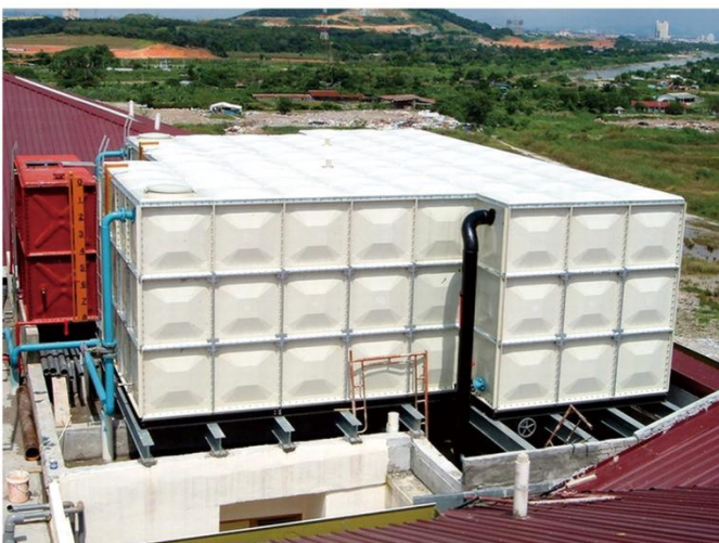
饮用水水箱 Drinking water tank
