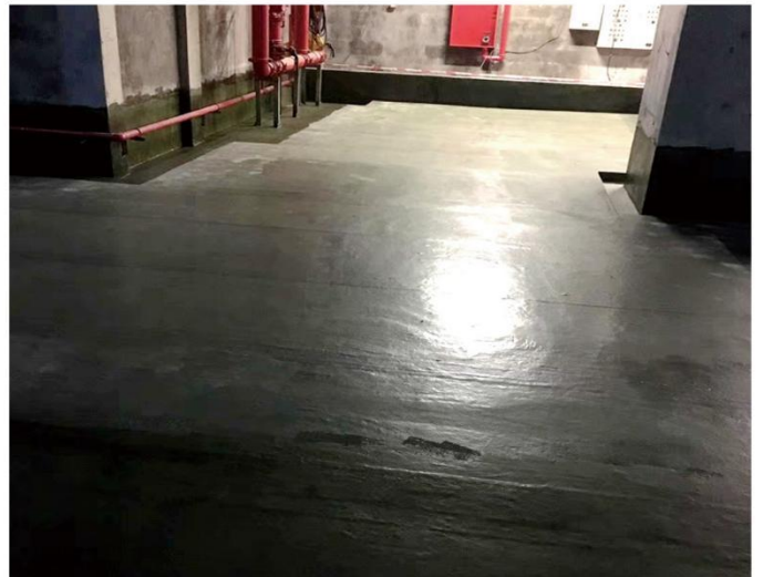
车间地面防腐玻璃钢 Shop floor anticorrosive FRP
