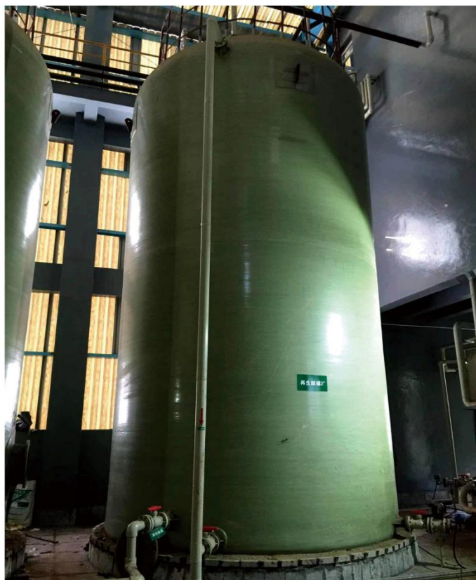
漂洗罐 Rinsing tank
