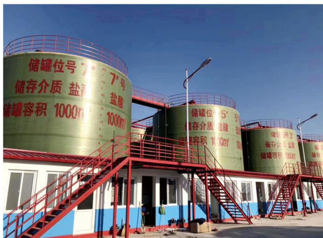
盐酸储罐 Hydrochloric acid tank
